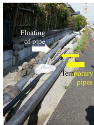
Fig. 10. Floating damage of water pipeline in Itako City
