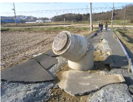
Fig. 11. Backfill liquefaction effects on embedded pipeline; note that no liquefaction happened in the farm land (Naganuma City in Fukushima)
