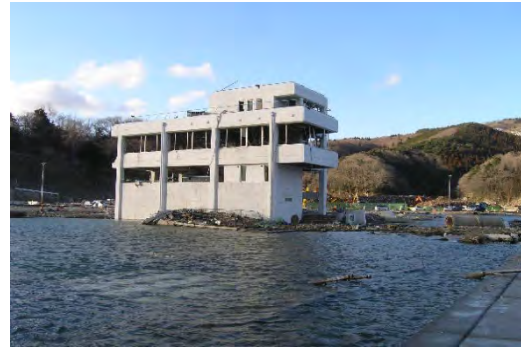
Fig. 26. Tectonic subsidence in Onagawa Harbor near Sendai where ground level is lower than the previous level by more than one meter
