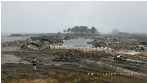
Fig. 5. Damaged seawall near the Abukuma River mouth
