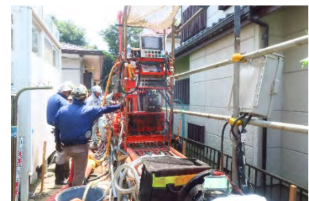
Fig. 22. Ongoing ground improvement by small jet grouting device in a very narrow space among houses
