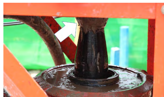
Fig. 20. Hindrance of jet grouting by unforeseen buried plastic drain
