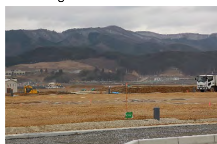
Fig. 24. Vast size of elevated ground in Rikuzen-Takata City
