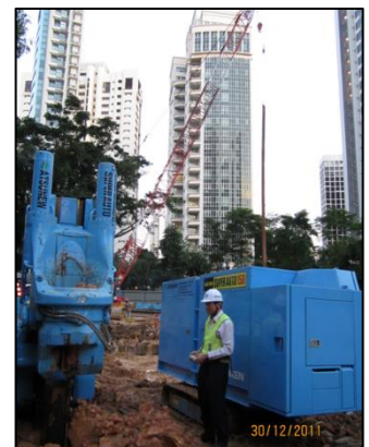
Picture 6 Power source of construction site
