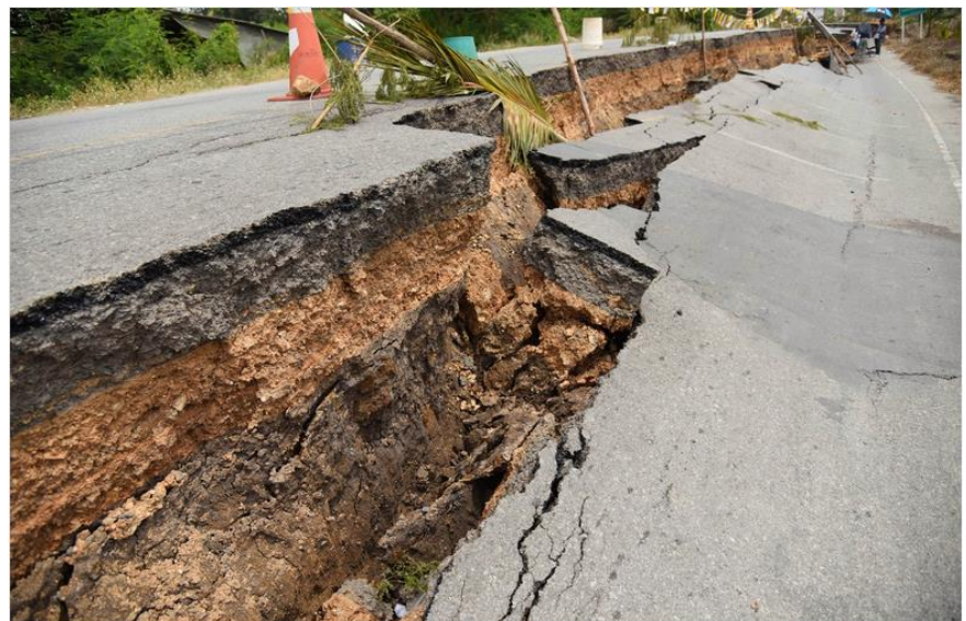
Photo 1 Road settlement alongside of irrigation area canal
