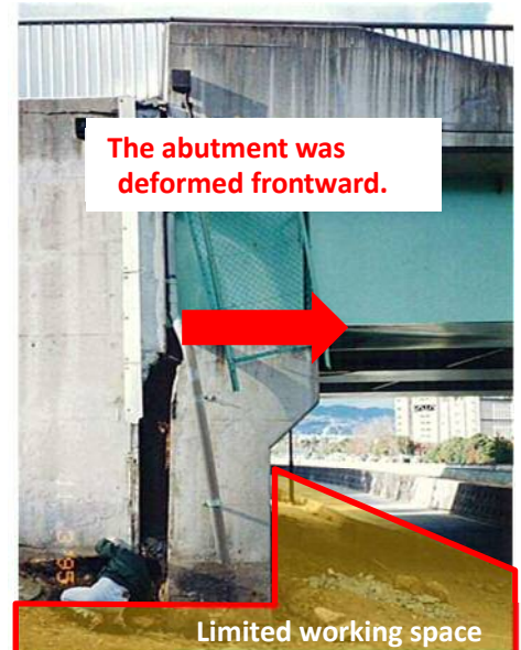
Fig. 6 Example of structure damaged by lateral movement due to liquefaction of ground
