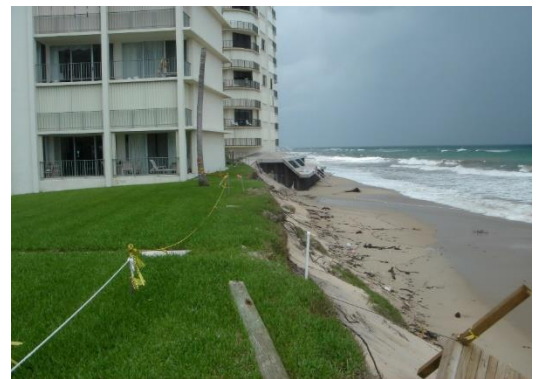
Fig. 2. Beach Erosion at Singer Island, Florida (2006)
