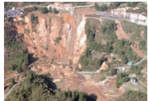
Photo 1.6 Landslide at Former Yamakoshi Village 9)
