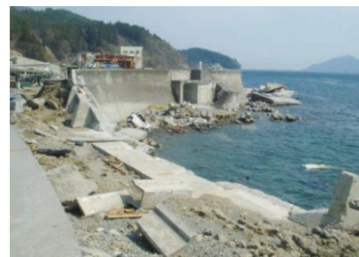
Photo 1.8 Seawall damage at Sanriku Town, Ofunato city 10)
