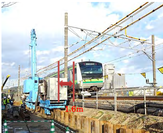
Picture2: Non-staging system (outbound line)
