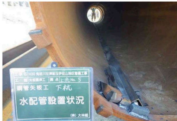
Photo 3. Internal pipeline for water supply.
