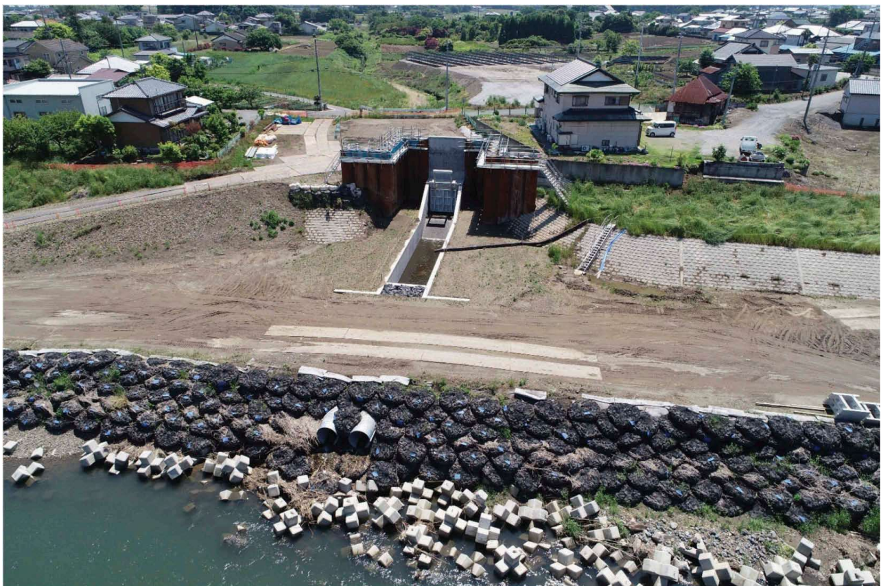
Photo 13. Completion after providing with the flap gate at the center of the pile wall.
