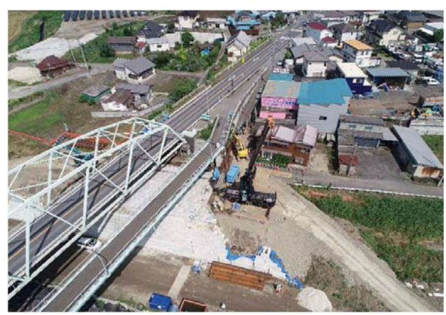
Photo 11. The Zero Piler used for sheet piling adjacent to the abutment structure.
