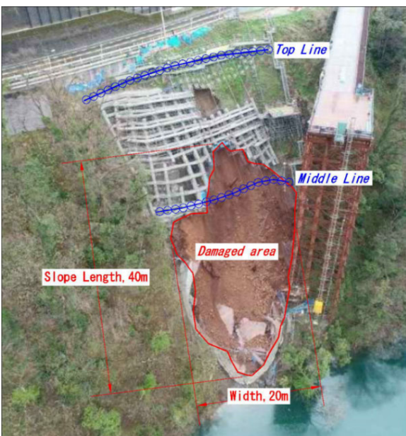
Figure 3. Status of damage [1]
