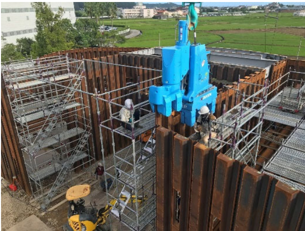
Fig. 31 Steel sheet pile press-in (piling work at GL+8m height with SILENT PILER™)
