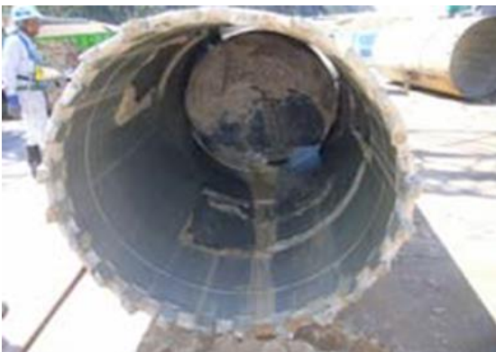
Photo 9. Inner blockage of casing by boulder
