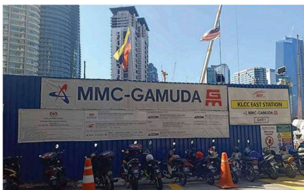
Figure 12. One of the construction site for mass railway Transit in Kuala Lumpur (Yun, 2020).
