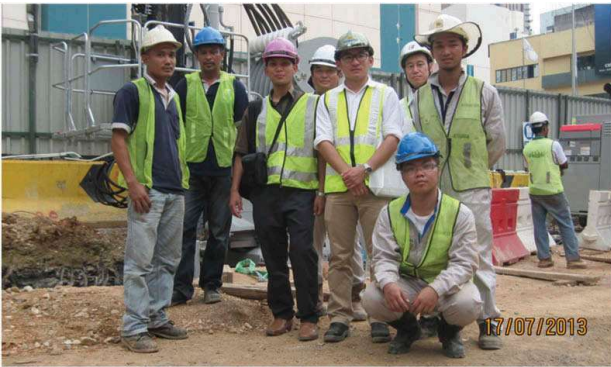
Figure 32. A site visit at MRT construction in early 2013 utilizing a crush piler machine for the first time.
