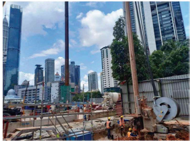
Figure 16. Lifting and transferring sheet pile to the crush piler by using crane machine (Yun, 2020).
