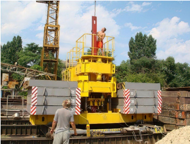
Figure 1. General view of hydraulic pressing equipment (full-scale testing device)
