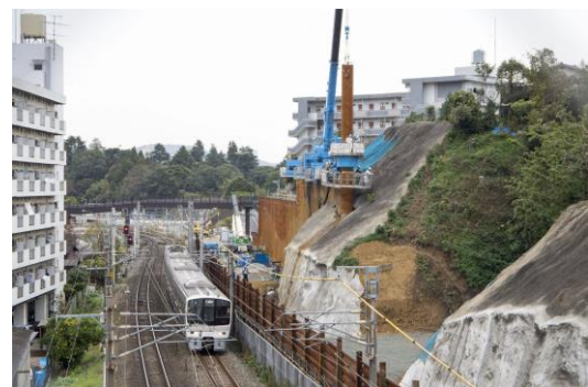
Fig. 1 A case study of the installation (Seki et al., 2016)
