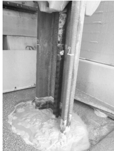
Fig. 12 Image taken during site testing showing silt particles suspended in water rising from the piling borehole
