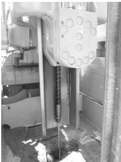
Fig. 11 Image taken during site testing showing a clean and polished pile on extraction of test No.21
