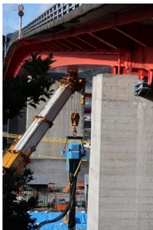
Photo 2. Planned augers and casings and an increase in the number of supervisors enabled the piling operation.
