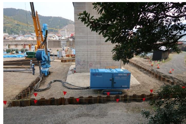
Photo 4. For the enclosure with closed corner, the piling operation was being conducted carefully after the installation under the bridge.
