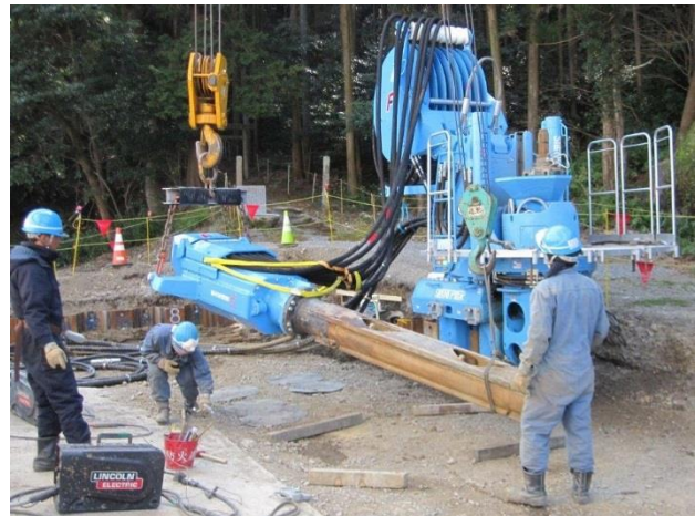
Photo 3. Mutual hoisting with the 4.9ton telescopic crawler and 50ton rough terrain crane, when the Pile auger is laid on the ground
