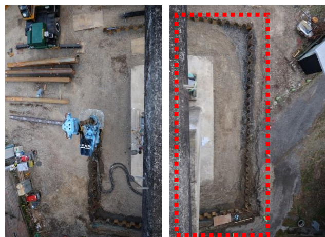
Photo 5. Setting up the 50ton terrain crane could not be set at the location inside the dashed line, where the ground was narrow and possessed differential elevations. Press-in operation was carried out by the F111 only, without the crane support to lift the Pile auger.
