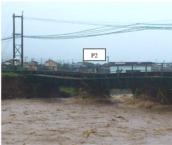
Fig. 2 View during the flood
