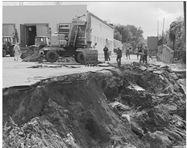
Photo 4. Landslide in Dnipro-city
