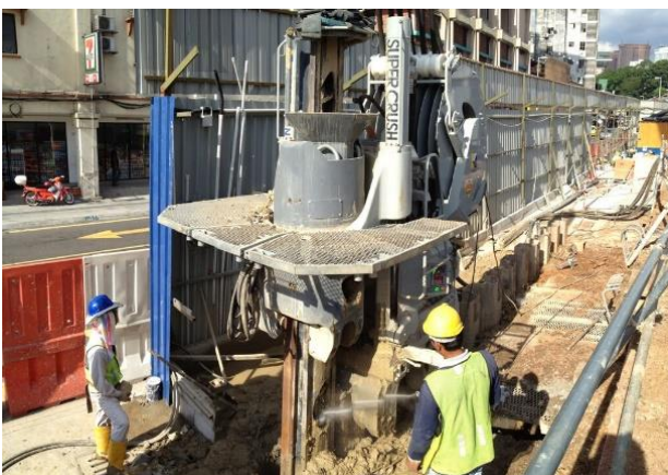
Fig. 1 Sheet pile installed by Super Crush Piler for MRT construction at Pasar Seni MRT Station
